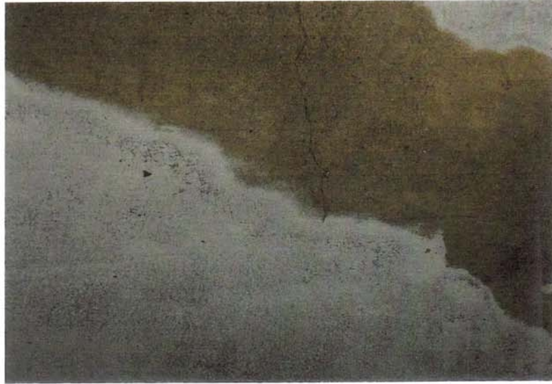
FIGURE 6: High Stress Area at Level 1, Willis Street Showing: - crack and its bridging by membrane - removal of membrane but no delamination
