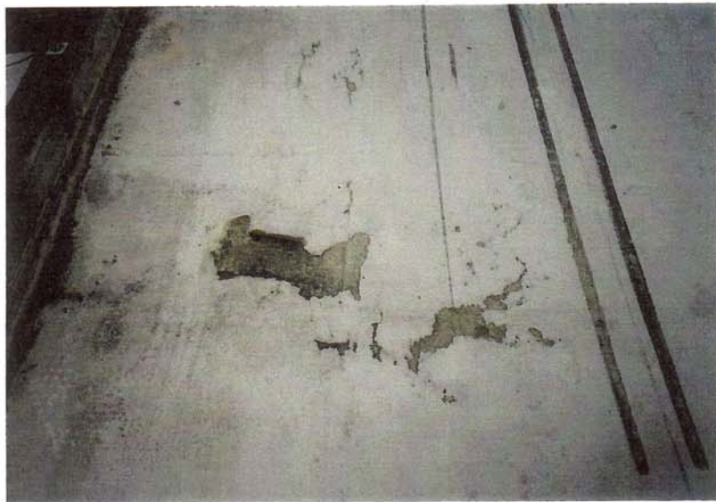
FIGURE 7: Delamination in Localised Area of Water Ingress
