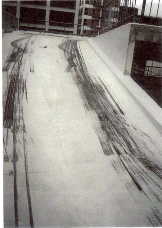
FIGURE 5: Ramp (Willis Street) Showing Blackening and Wheel Spin Areas
