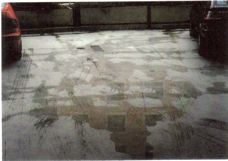
FIGURE 2: First Level Deck, Digital House (beige colouring is reflection of adjacent building in the surface water)
